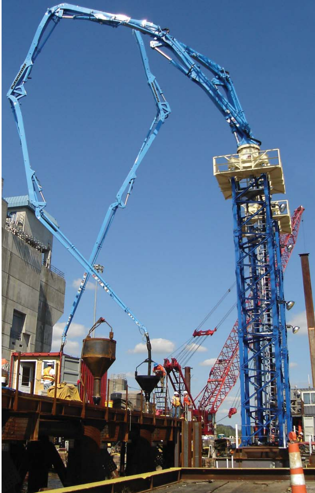
The two Putzmeister MX 43/47Z placing booms, the industry's largest that do not require counterweights, deliver concrete to the tremie pipes which move it underwater to its final destination.
