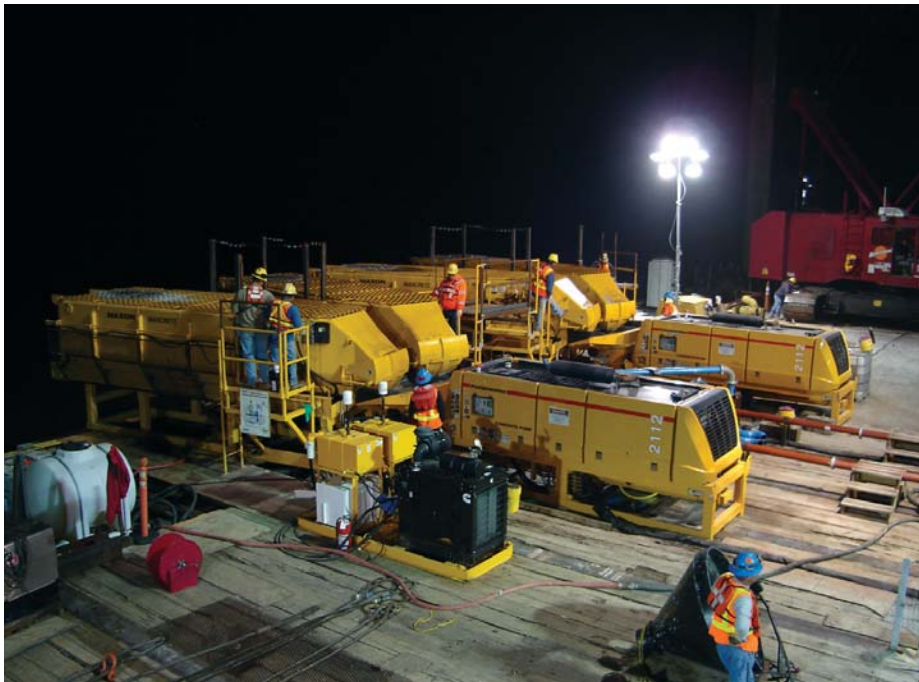
The placement of the concrete for each of the 28 shells is a non-stop 36-hour process.
