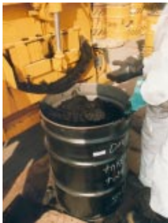
Left: A two (2) cubic yard capacity Mini-Maxcrete, with hydraulic discharge gate, feeds mixed sludge to 55 gallon drums for disposal.
