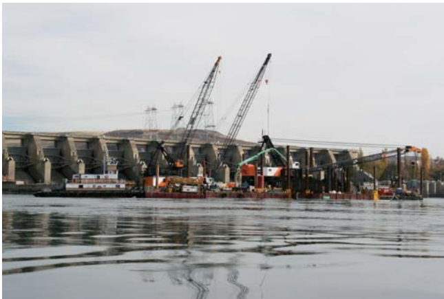
Barge mounted concrete production equipment - Maxon Maxcrete feeds trailer pump, and 32 meter placing boom
