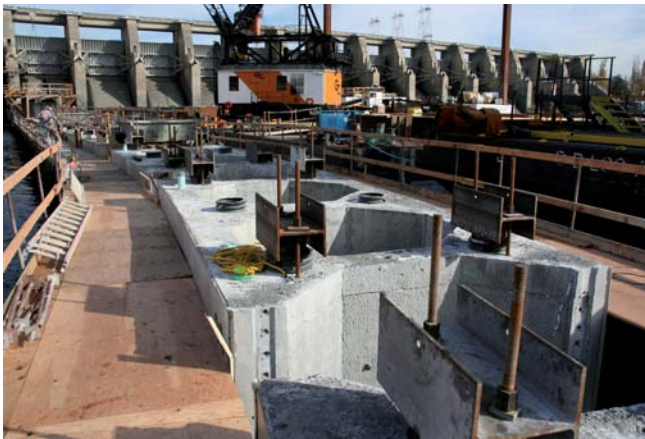
Top of precast section visible above the water line are tied into rut slabs below
