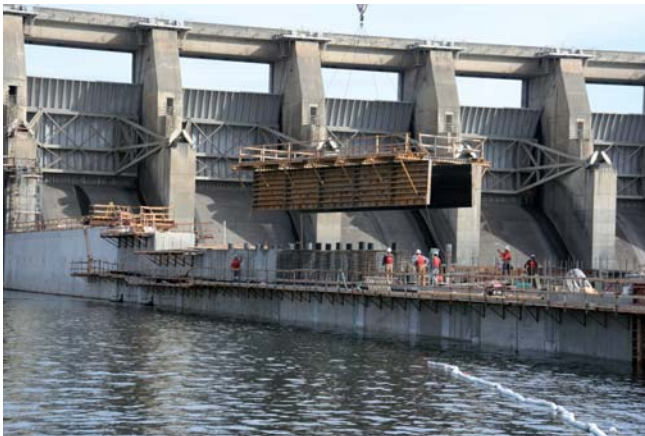
Precast caps are lowered into place during the final stages of the wall construction.
