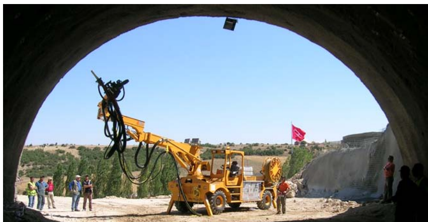
Putzmeister WetKret 5 self-propelled robotic shotcrete unit, complete with pump, air compressor, dosing pump and telescoping articulated 54' vertical reach.
