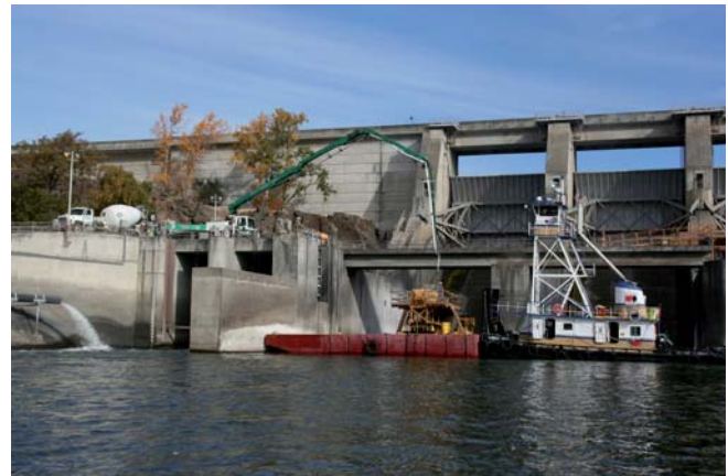
9 cubic yard truck mixers and 32 meter concrete boom truck feed concrete to barge mounted Maxcrete
