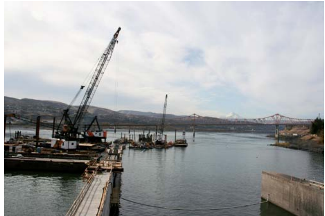
(View looking down stream): Shorter Spillway Wall 5/6, built in 2004, is shown in foreground at right, new 830-foot Spillway Wall 8/9 extends downstream from the dam at left, in the final stages of construction (snow covered Mount Hood visible on the horizon)
