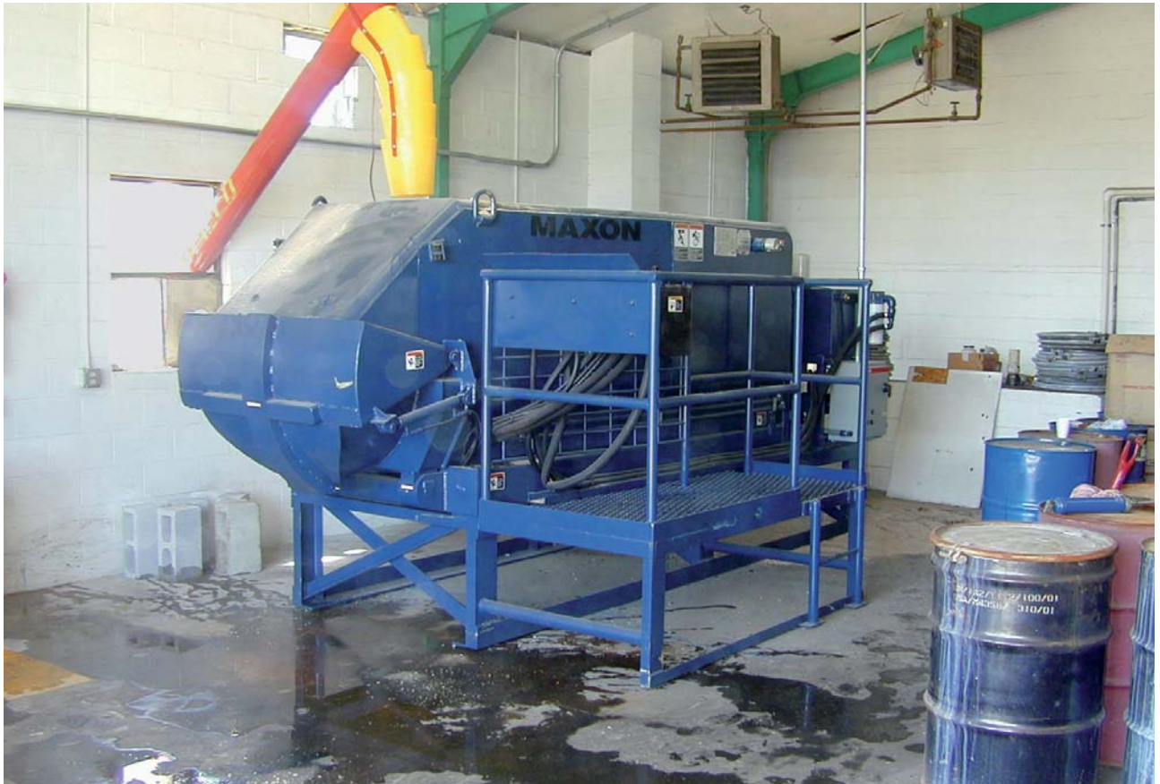
MAXPRO SPU 4.5 Pharmaceutical Waste processing system. In plant installation complete with elevated platform for direct discharge to 55 gallon barrels. System also included a cement silo (located outside the building) with screw auger feed for dustless charging of MAXPRO with solidification agents.
